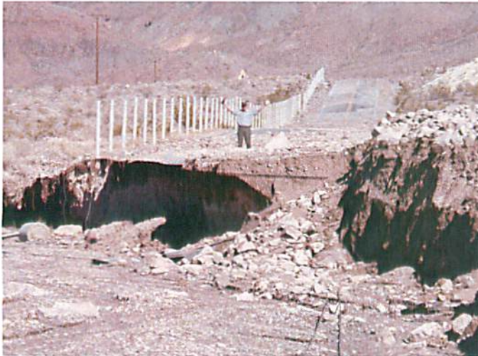
Large sections of Scotty's Castle Road and historic fencing were destroyed.
