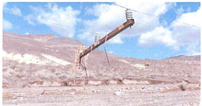
24 power poles that supplied electricity to Scotty's Castle were washed away.
