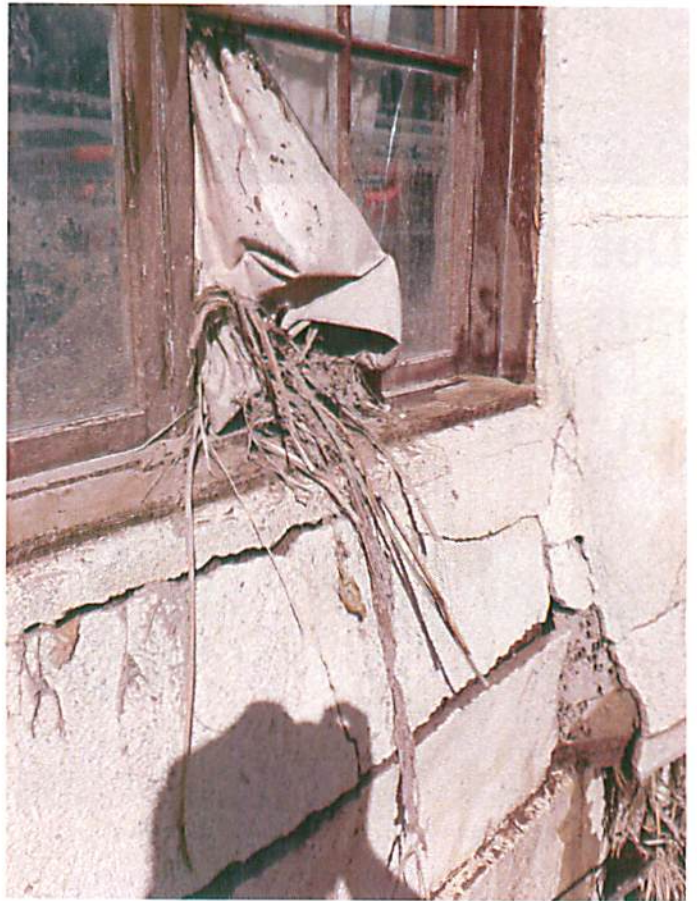
The Visitor Center's south wall was punched out by the force of the flood inside the building. Another section of exterior wall was pushed 18 inches off the foundation.
